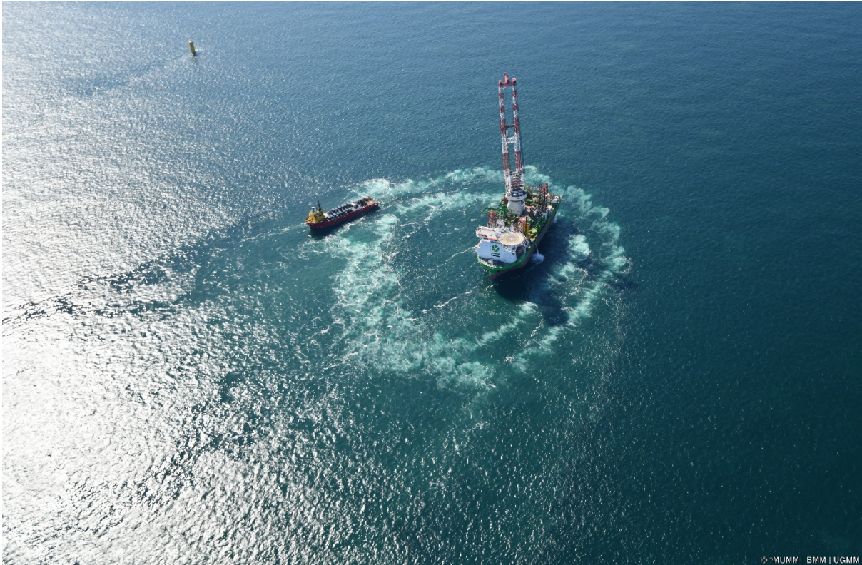
Monitoring of construction activities in the wind farms: the use of a bubble curtain during piling activity. © RBINS/UGMM
