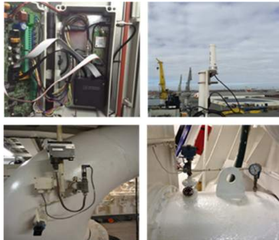
Figure 3: An installed EMS 2.0 system and its sensors
